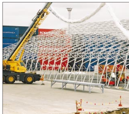
After the frame is erected the cover is lifted onto the frame.
