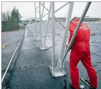
Frame elements are arranged at the hall location and fastened together into frame sections with bolted joints.
