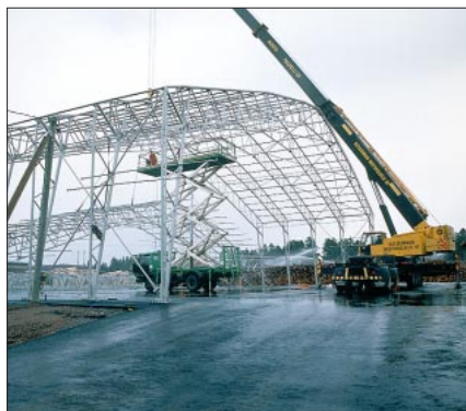
The frame is raised one section at a time and the sections joined together.
